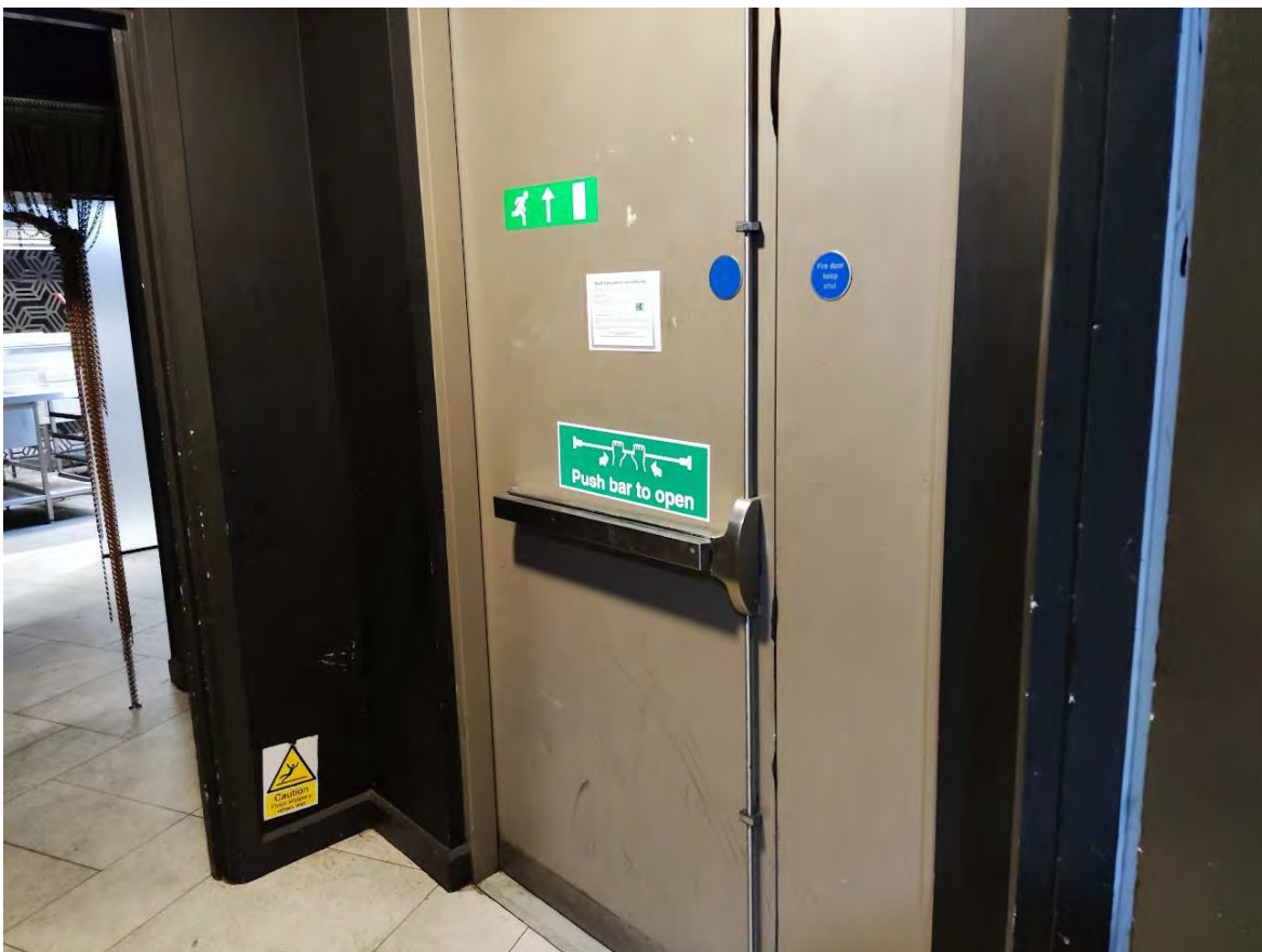
Figure 7: Fire-doors are robust metal construction
